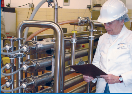
Membrane filtration equipment at the WCDR.
